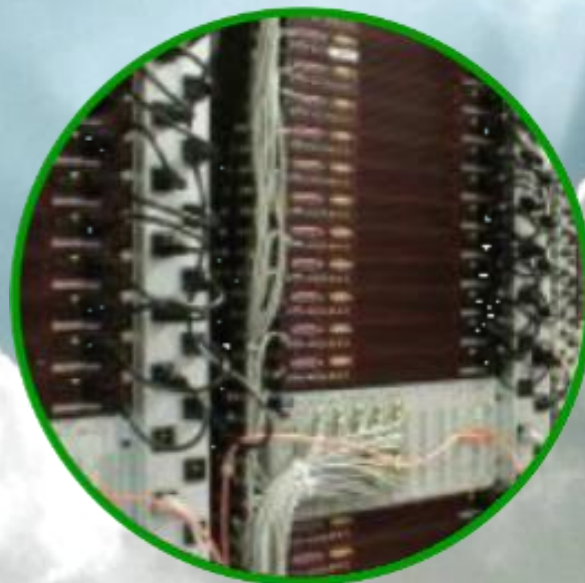
Purpose built hardware
